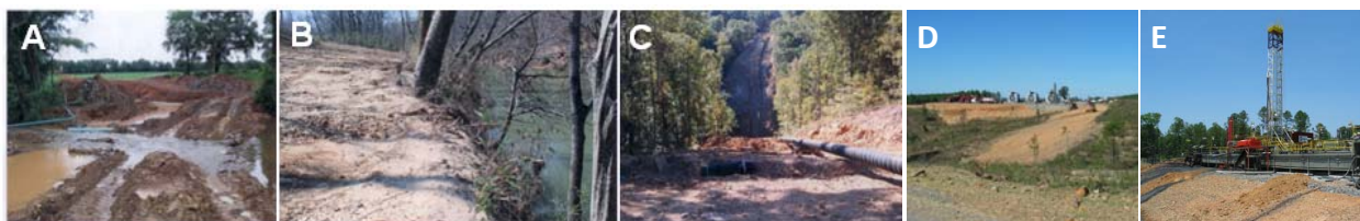
Fig. 1. Sedimentation from installation and maintenance of natural gas wells. A) Stream trenching for laying pipe under a small stream; b) ditch and fill activities along the riparian corridor of a stream; and C) slope clearing of vegetation to lay pipe for gas distribution, D) compressor sites, roads, and E) gas wells. Photos courtesy of Lindsey Lewis, USFWS
